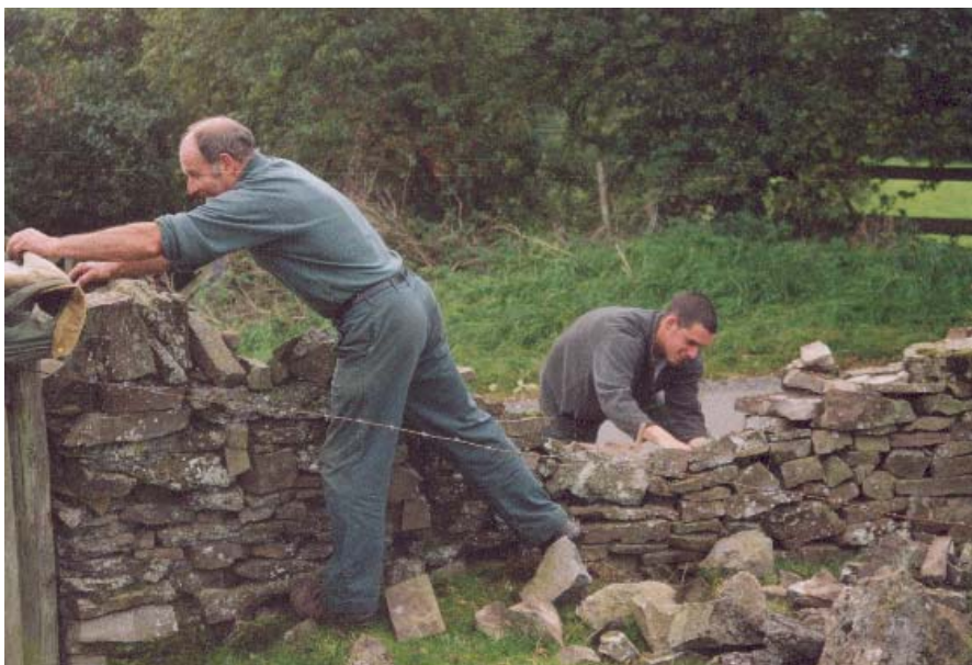
Dave & Robert Marpole, local walling experts, work on one of the walls in Norbury Village.
